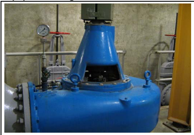
Raw Sewage Pump 3
