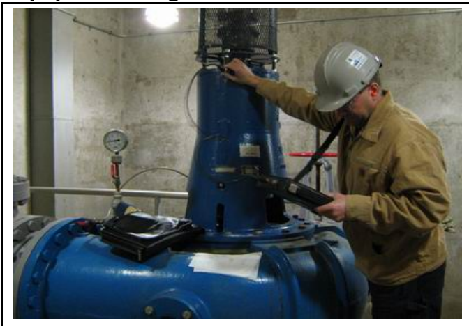
Raw Sewage Pump 1
